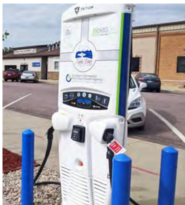
SMMPA's DC Fast Charger in Saint Peter
