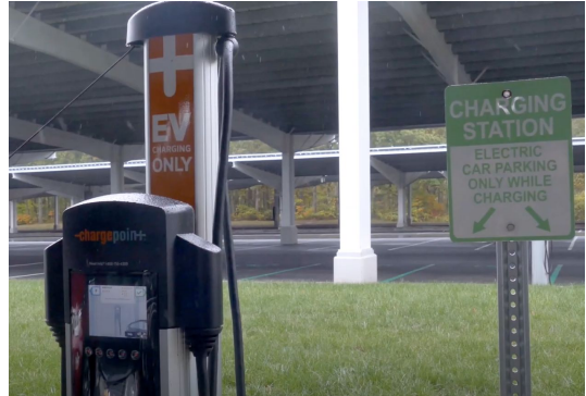
Bristol Community College's Charging Infrastructure
