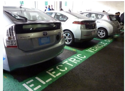
BU's Charging Infrastructure
